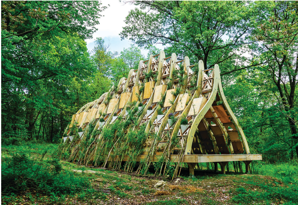
The architects anticipate removing the scaffolding and completing the interior for independent human use within five years or less. Photo courtesy the architects.
